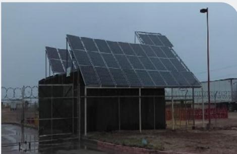
Solar panels installed atop our organic garden
