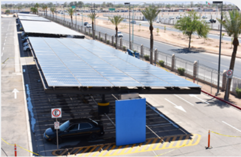
Solar panels installed as part of our 'Carport project' in our Mexicali plant (SPMX1)
