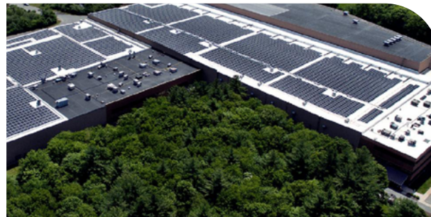
Performance Line Solar Panels Rooftop Installations
