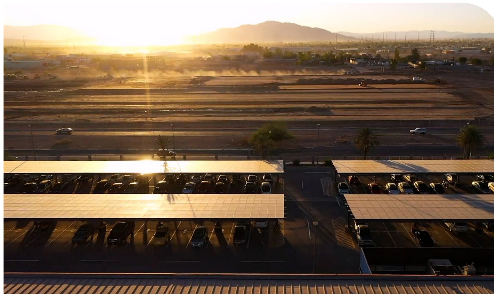
Carport solar in Mexicali, Mexico facility
